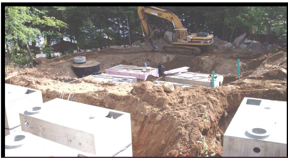
PROCTOR BACKWASH EFFLUENT TREATMENT
